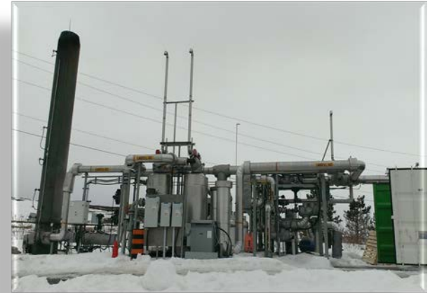
Landfill gas collection system at Walker Environmental in Niagara is used for WTE
